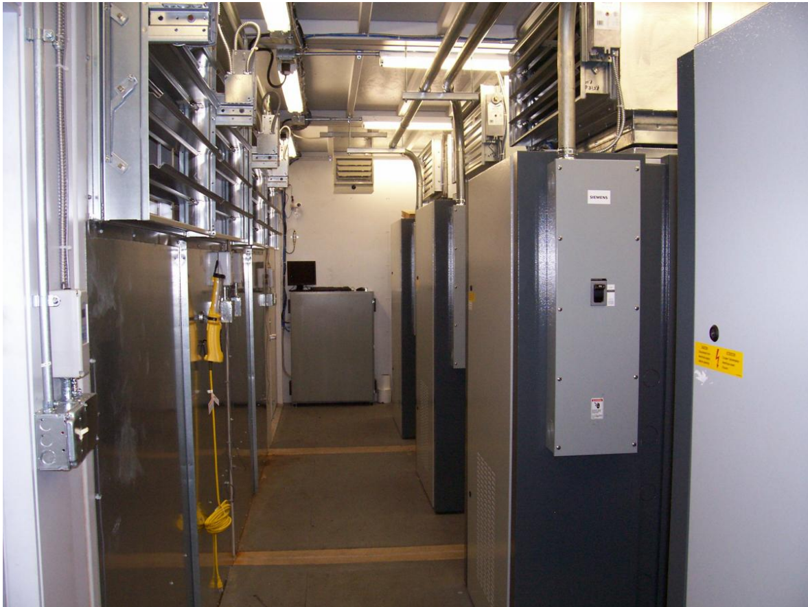
The DirectAIR® Compressed Air Facility
