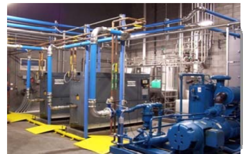
After Transair installation First year savings $38K
